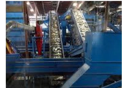
Materials Recovery Facility (MRF)
