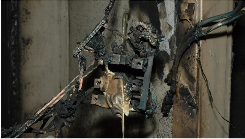
Typical damage from bypassing the meter
