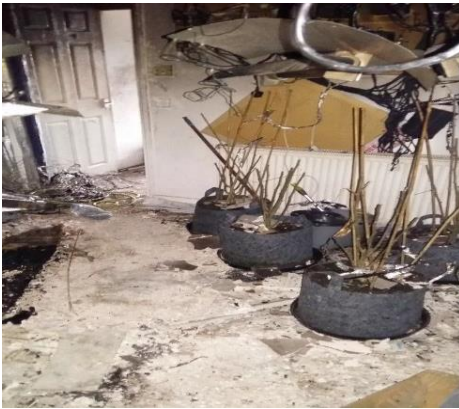
Cannabis plants and equipment on ground floor
