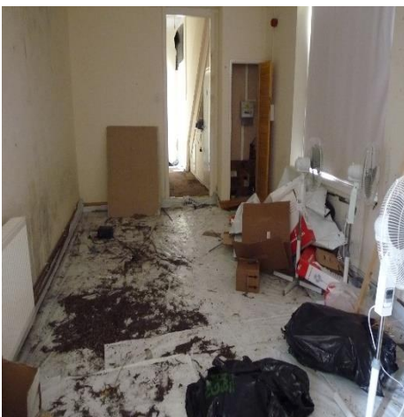
Condensation has resulted in significant spoiling of decorations
