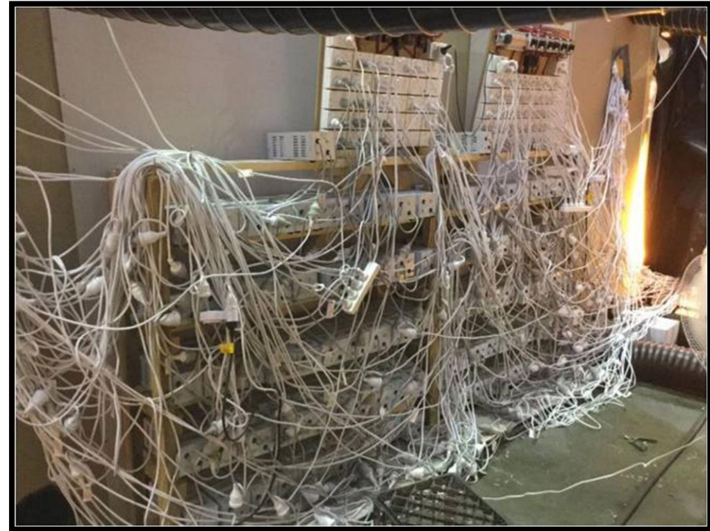
Complex distribution of electricity stolen directly from a substation
