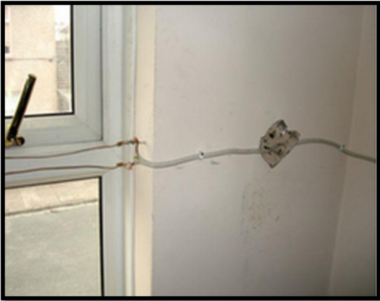
Window fittings wired to the mains
